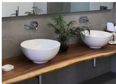
Encimera de madera tropical y lavabos redondos modelo Lounge Tropical Wood sink counter with round wash basin.
